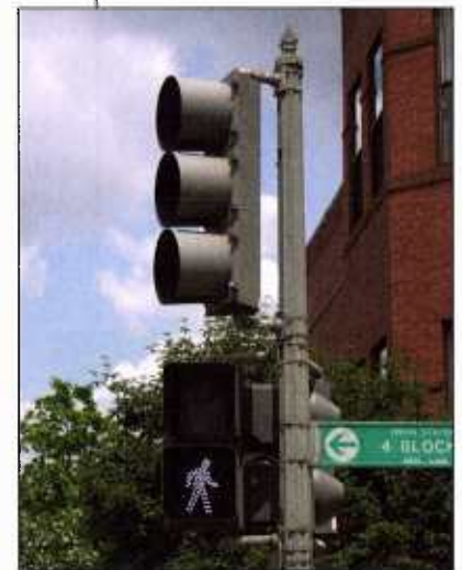
Exhibit 4-4. Vehicular Signal Heads Are Obscured So Pedestrian Signals Are Necessary.
